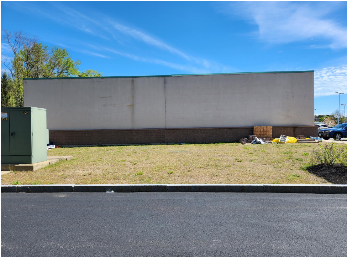
P3: AREA OF ADDITON FROM A WEST TO EAST POINT OF VIEW.
