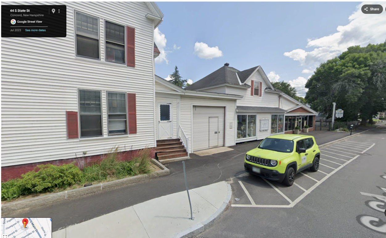
Existing Overhead Door to interior loading area (view looking south). Sidewalk tip downs and "No parking" striping are existing.
