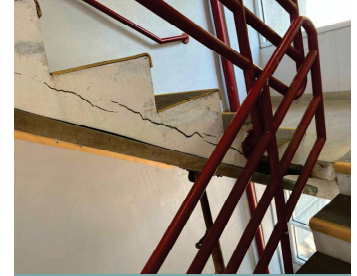
Concrete splitting, original guardrail
