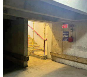
Lighted exit sign, original fire alarm devices
