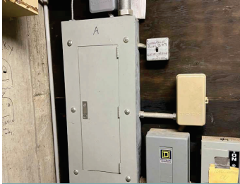
Basic electrical distribution, no lighting controls, no emergency power
