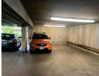
Linear fluorescent fixtures, embedded conduit
