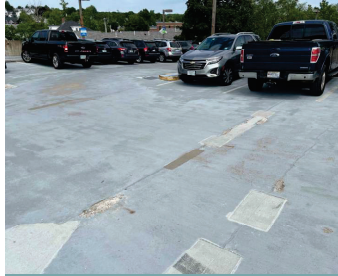
Previous slab repairs, cracking, delaminations
