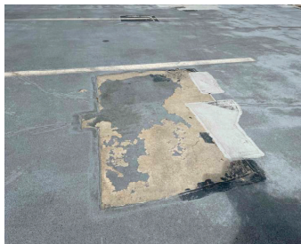
Deck coating debonded at previous patch
