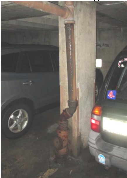
Figure 71 Firehouse Block Garage: 6” Sanitary Line Leaking at Connection at Upper Tee.
