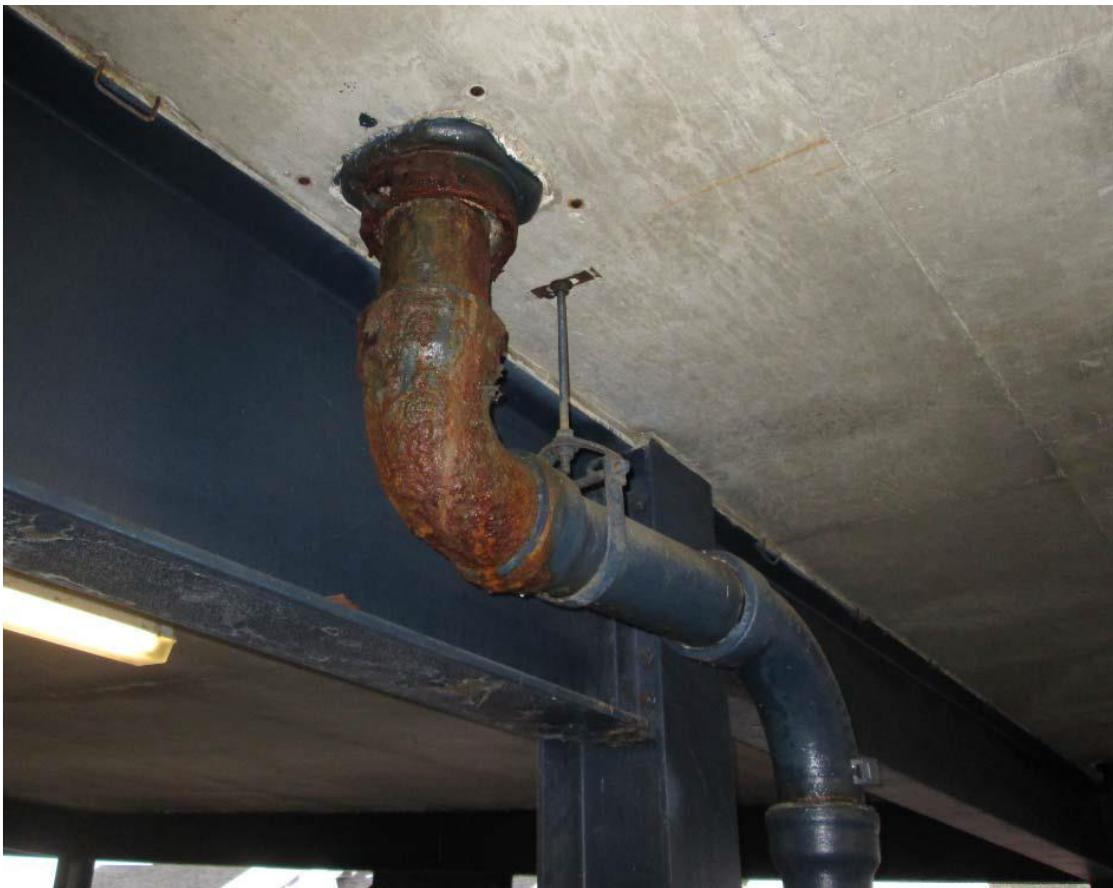
Figure 73 Durgin Garage: Negative Pitch and Corrosion of 6" Sanitary Riser at Column Line F4 Level 4
