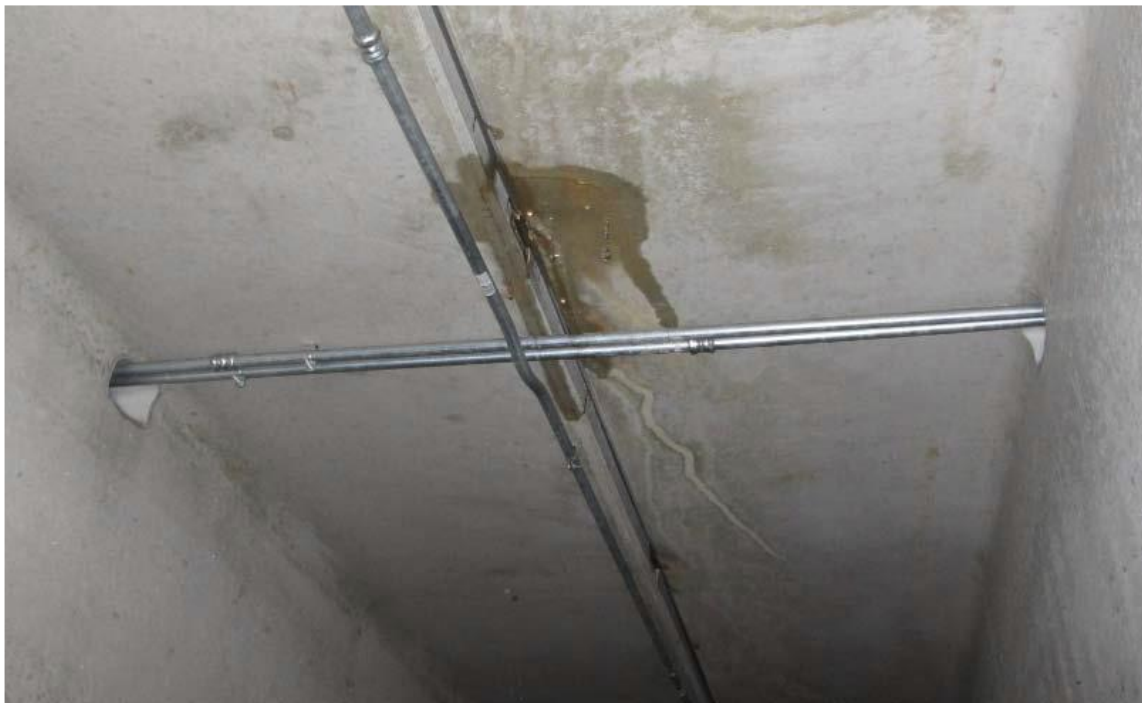
Figure 74 Capital commons Garage: Roof Leak Southwest Area
