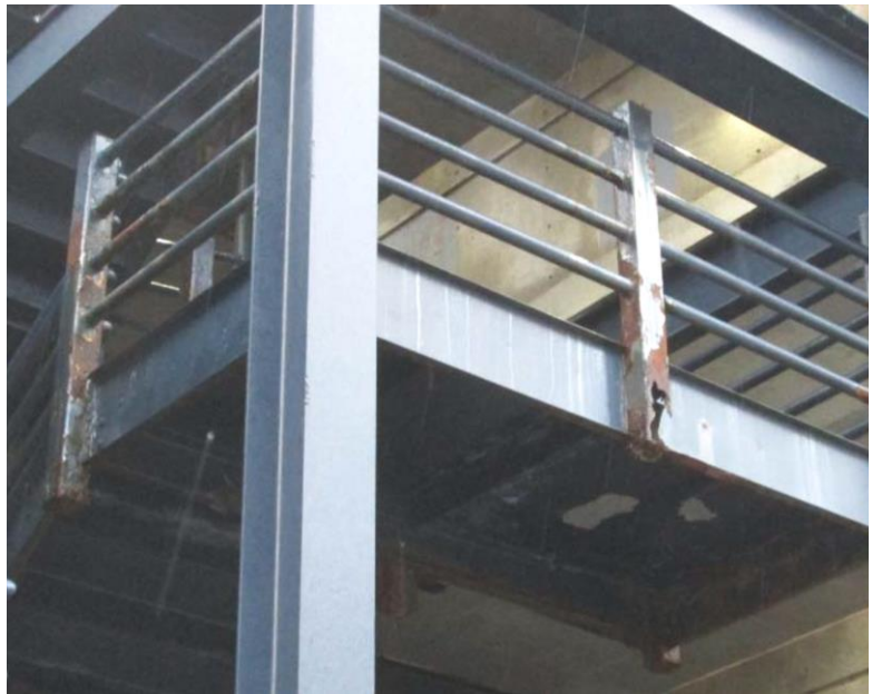
Figure 72 Durgin Garage: Rust and Decay in Metal Posts on Northeast Stair Tower
