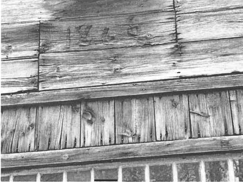
"1869," on the west end of the barn, and old glass in the transom window.
