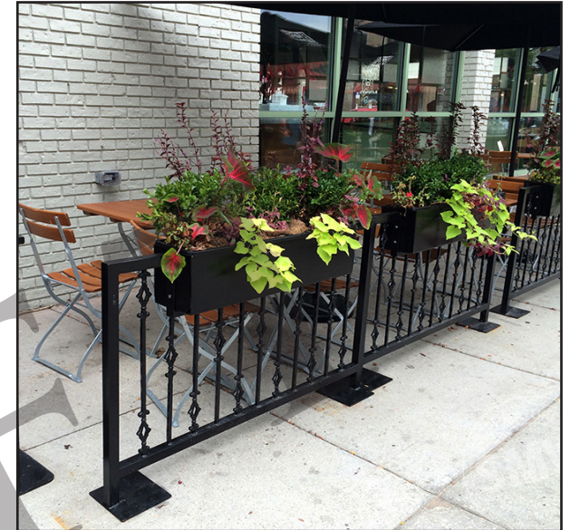
Outdoor dining enclosure utilizes quality materials, creates a sense of privacy with planters, has substantial base plates for stability, and takes up minimal space.
