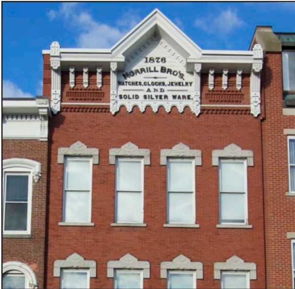
Prominently displayed building names, typically found near the cornice, can convey intriguing information about earlier occupants and uses.
