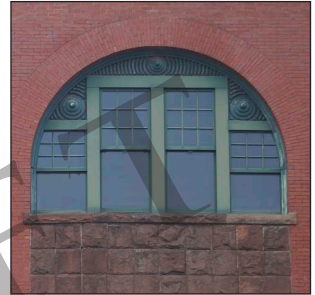
These replacement windows reflect the Queen Anne architectural style of the Chase Block.
