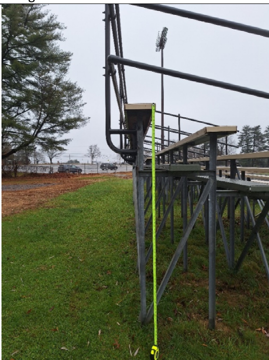
Photo 19: NFPA 102 5.5.7 Openings greater than 4".
