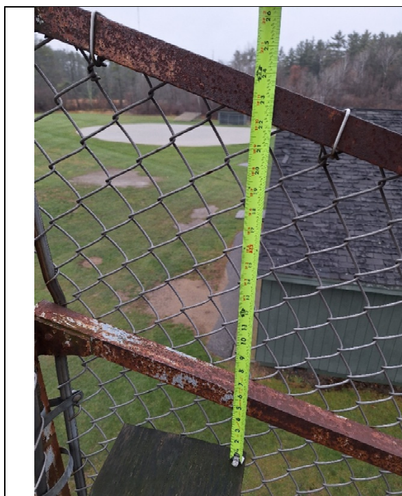
Photo 1: Railing is 24" from the top of the bench. NFPA 102 5.6.1 says no less than 36" from the center of the seat board and 42" from the floor board, typically all around.
