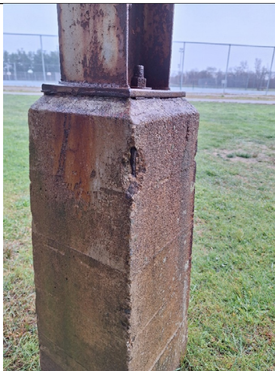
Photo 6: Rebar exposed in concrete pier.
