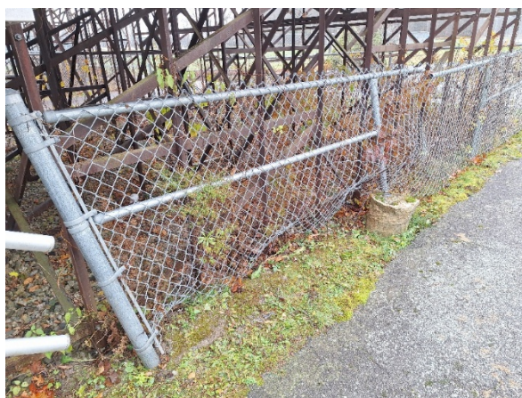
Photo 12 : Chain-link is broken and posts are loose in many places.
