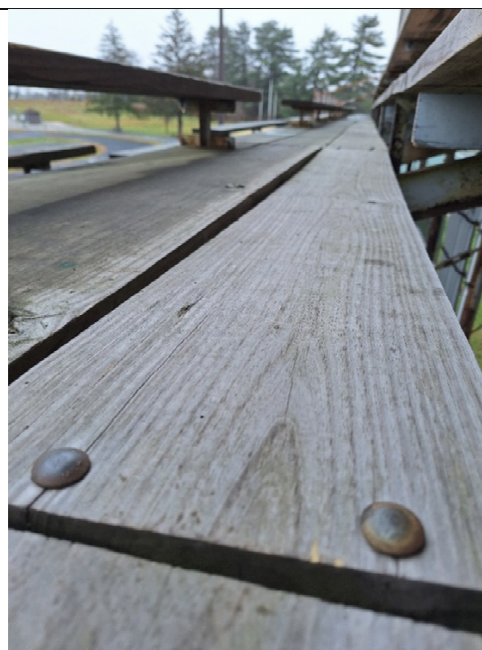
Photo 2: Wooden floorboards noticeably deflect.
