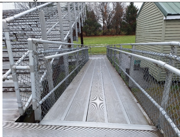
Photo 16: Ramp skews significantly to the right.
