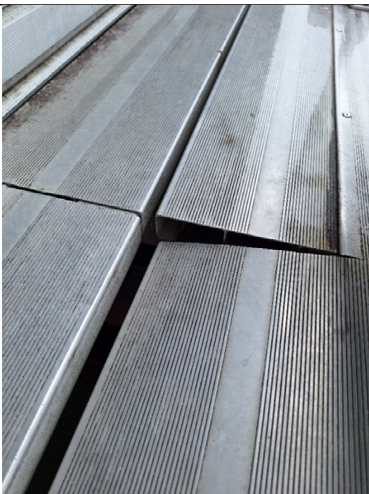
Photo 13: The metal floorboard is loose and deflecting. Occurs in multiple places.
