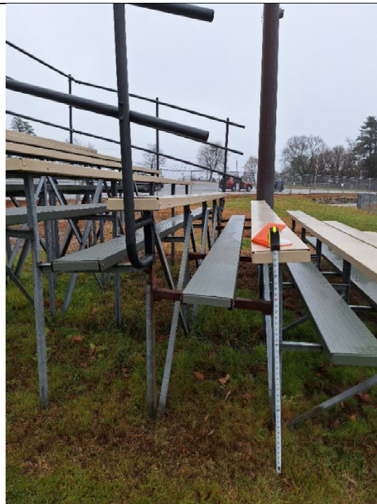
Photo 18: Railing does not extend low enough per NFPA 102 5.6.1.
