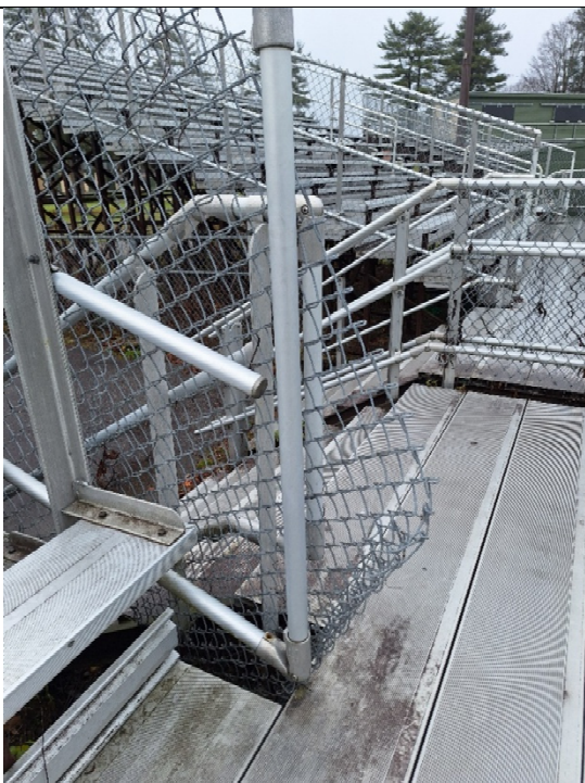
Photo 9 : Chain-link is loose and extending past vertical support.
