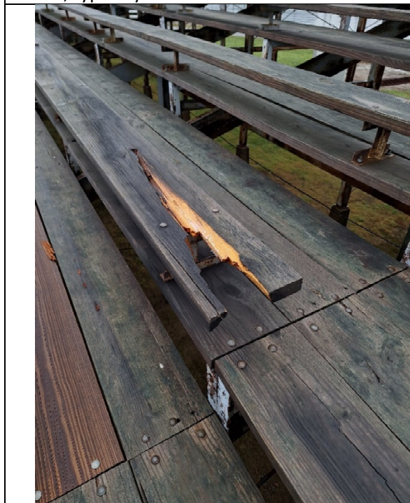
Photo 3: Broken wood bench.
