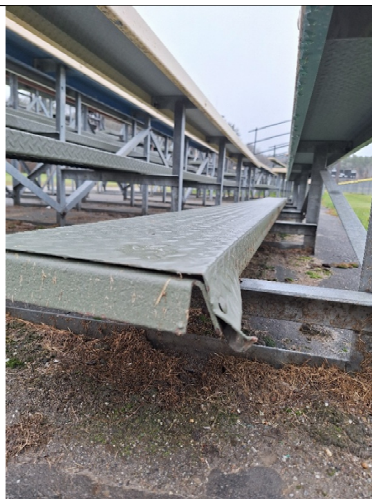
Photo 20: The edge of the floorboards and seating is loose or bent in many places.
