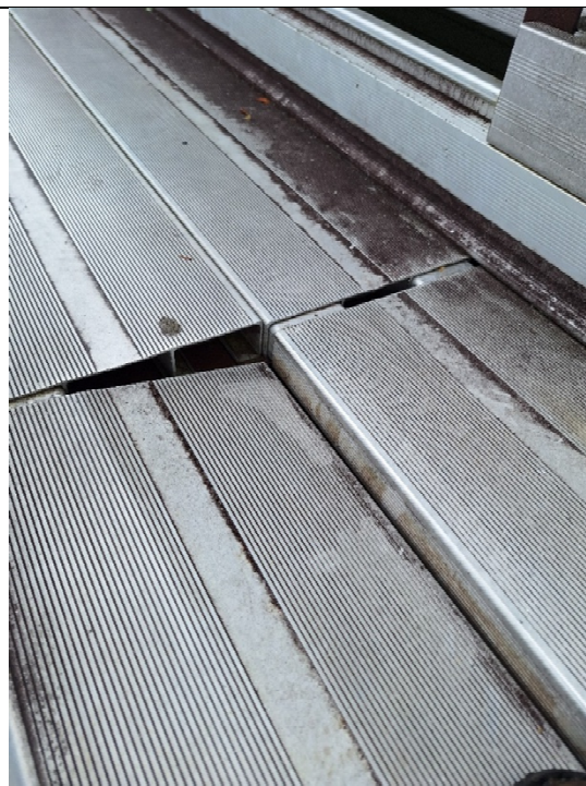
Photo 14: The metal floorboard is loose and deflecting.
