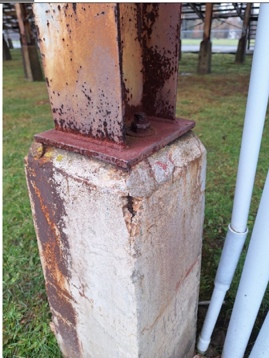
Photo 7: Rebar exposed in concrete pier.
