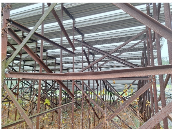
Photo 11 : X Bracing is bent in many places.
