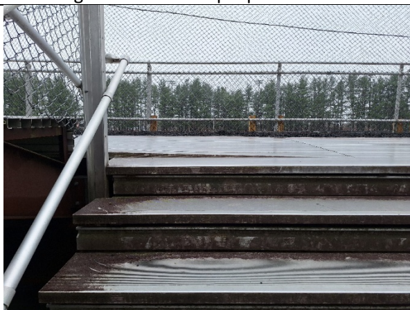
Photo 15: The top of the stairs does not align with the top of the decking.
