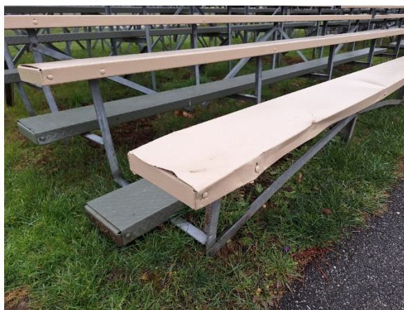
Photo 24 : Bent seating, typical in many places.
