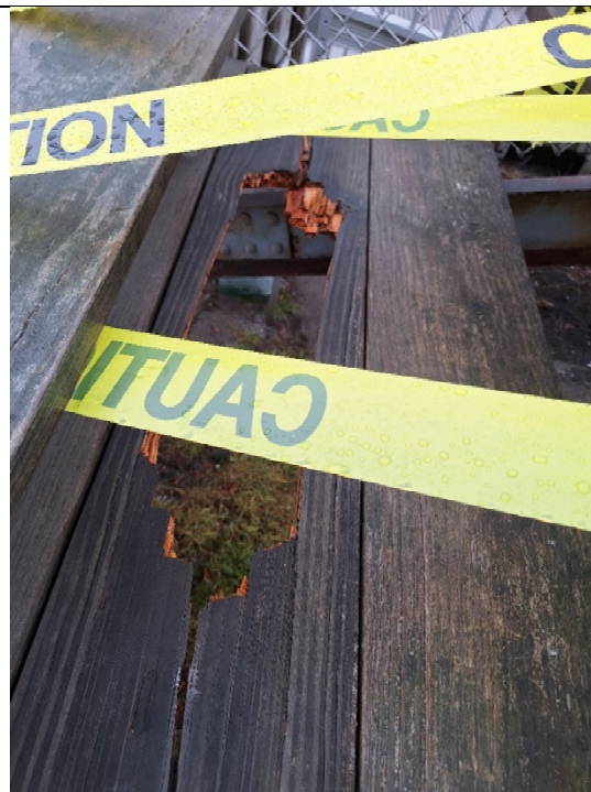
Photo 4: Broken wood footboard.
