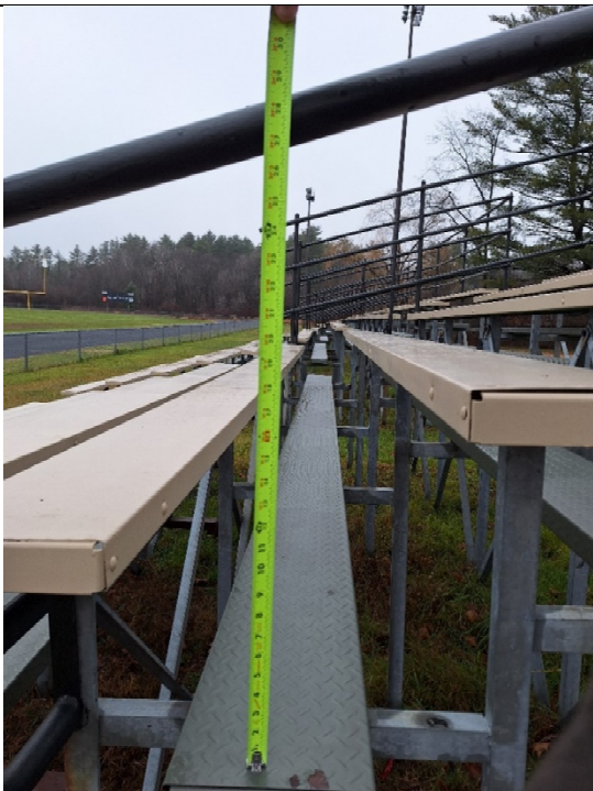
Photo 17: Opening larger than 4". NFPA 102 5.6.7 says no more than a 4" sphere can pass through the opening. NFPA 102 5.5.6 applies to the opening between the footboard and seats as well.
