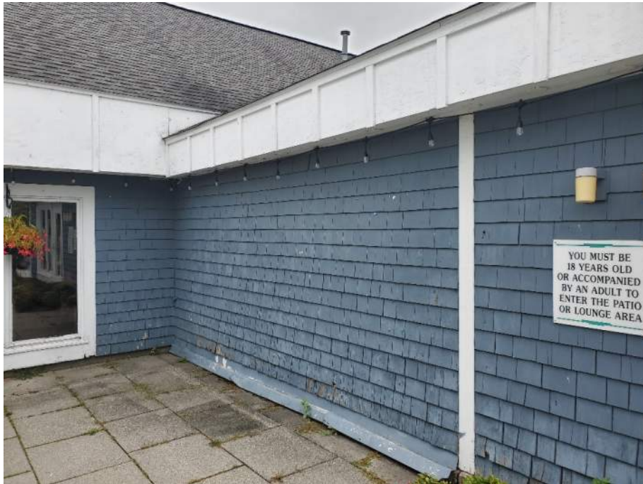
Damaged Siding & Roof Fascia
