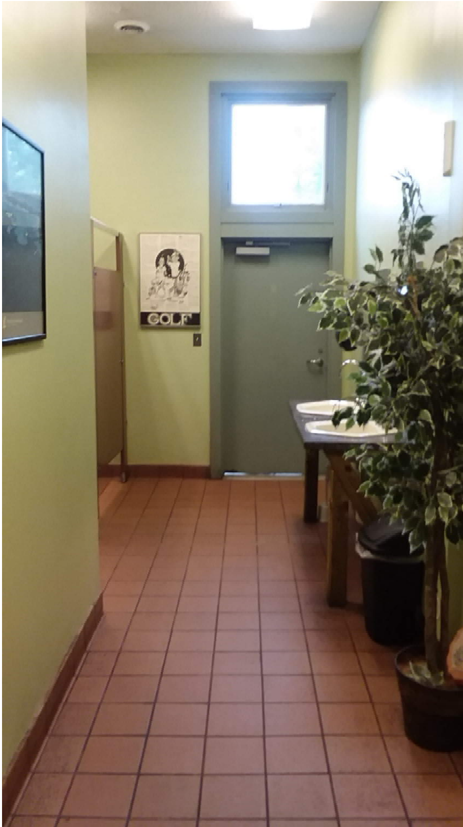
Exterior Door Threshold in Women's Restroom
