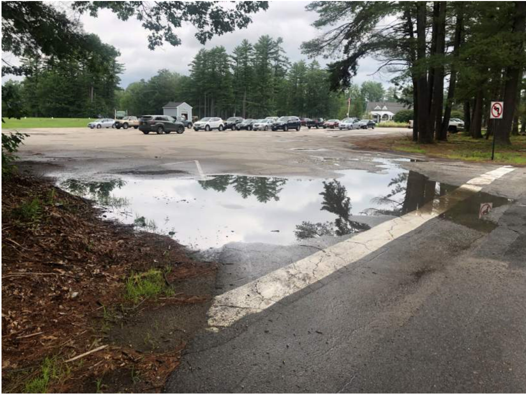
Significant Ponding – Parking Lot Exit onto Beaver Meadow Drive
