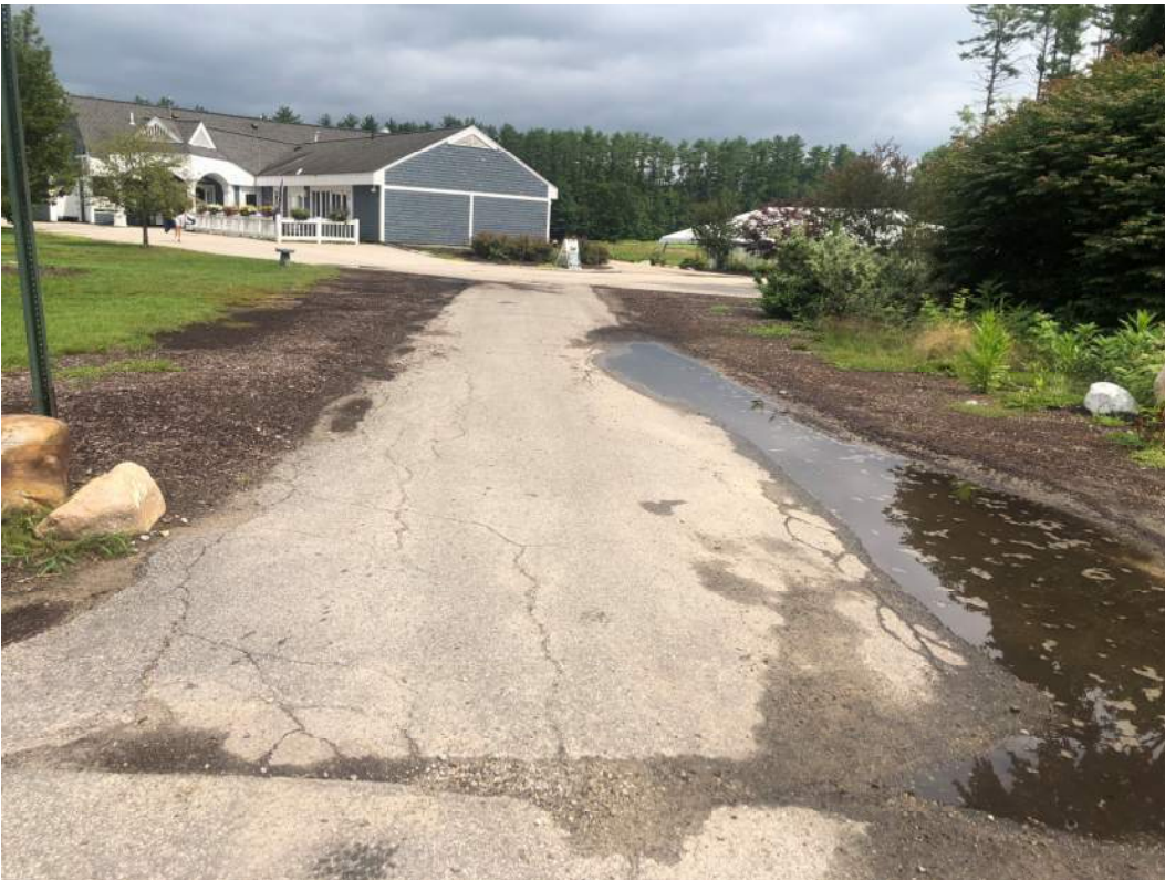
Ponding, Cracked Pavement and Collapsed Edges at Main Access Walk to Club House
