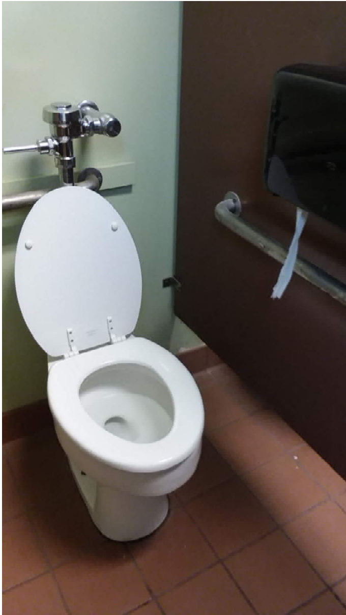
Missing Vertical Grab Bar & Non-compliant Rear Grab Bar Impairments
