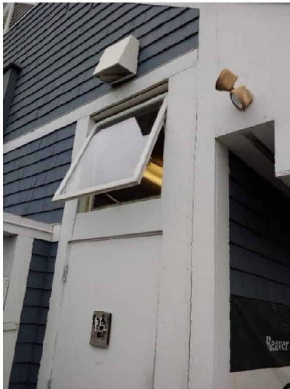
Incorrect Signs on Inaccessible Restroom Entrance
