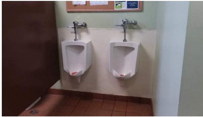
One Urinal Required to be Accessible when More Than One is Provided
