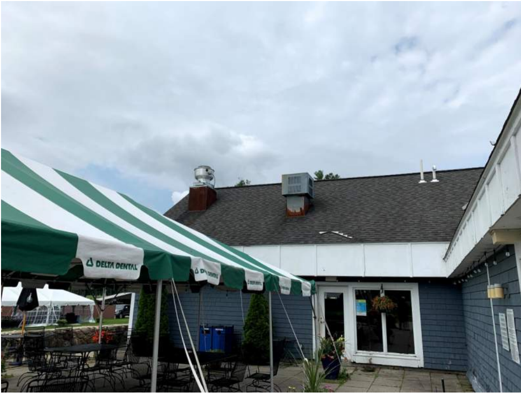
Intake and exhaust fan for kitchen hood
