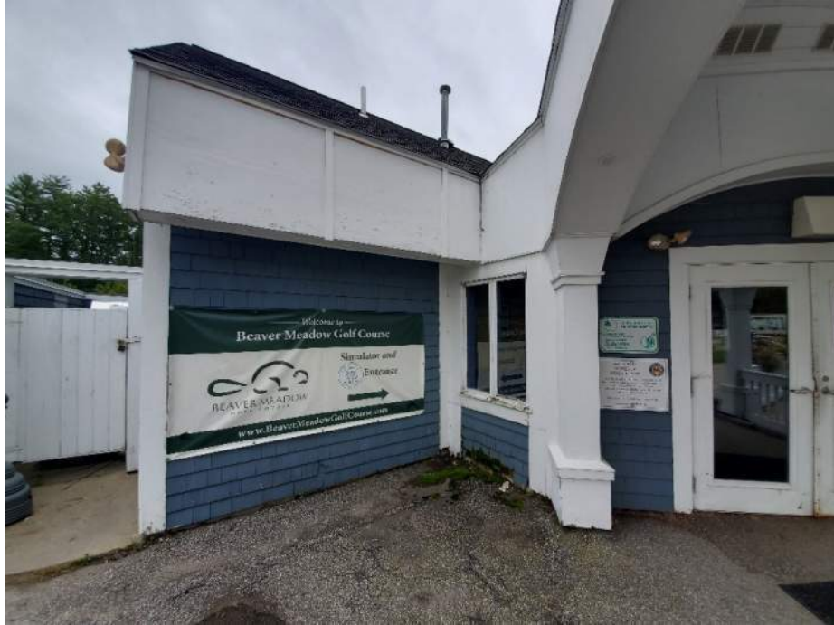
Damaged Siding on North Side
