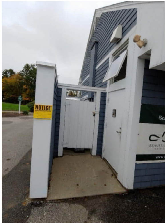
Public Restrooms Inaccessible from Exterior
