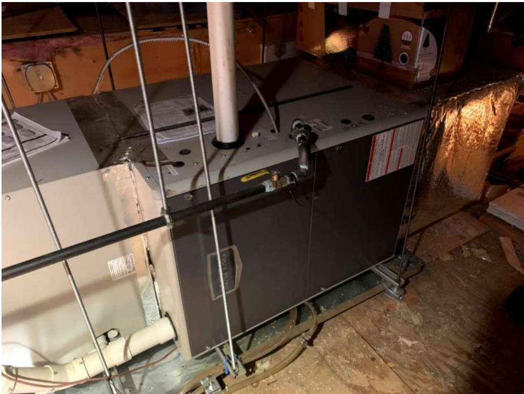
Bar/Pro Shop 5 ton air handler
