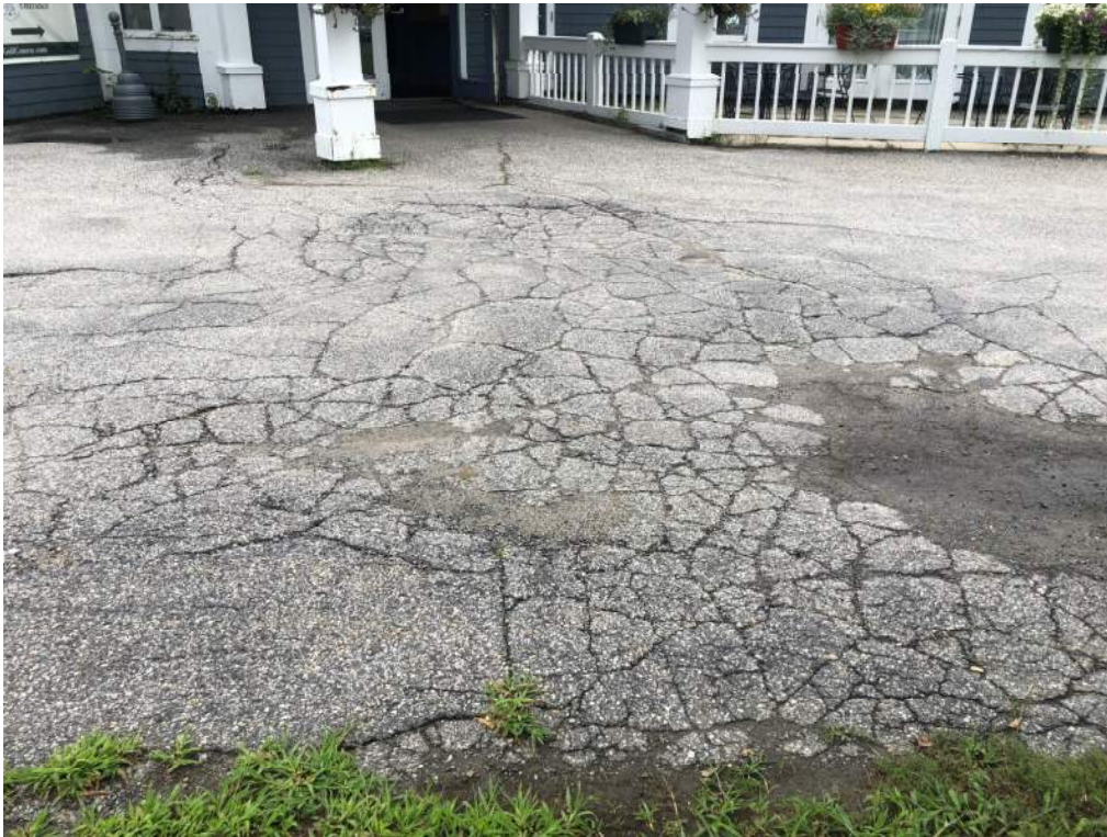
Badly Cracked and Deteriorated Pavement Located Near Main Entrance – North of Club House
