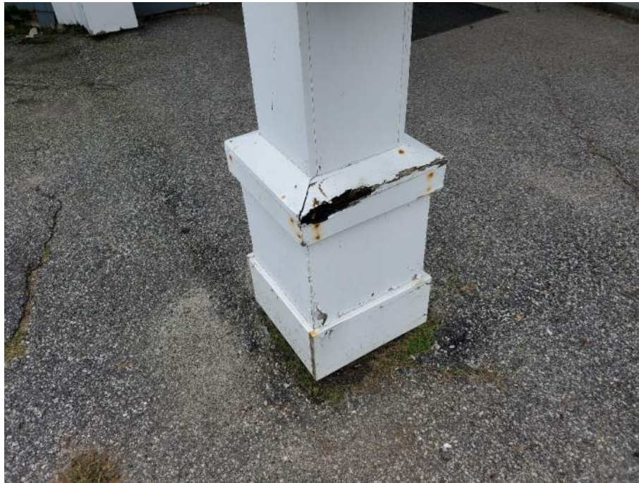
Rotted Trim at Column on North Side
