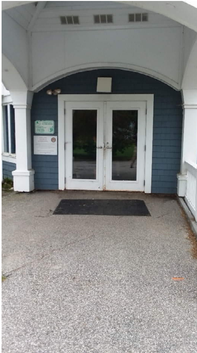
Accessible Entrance Sign Required
