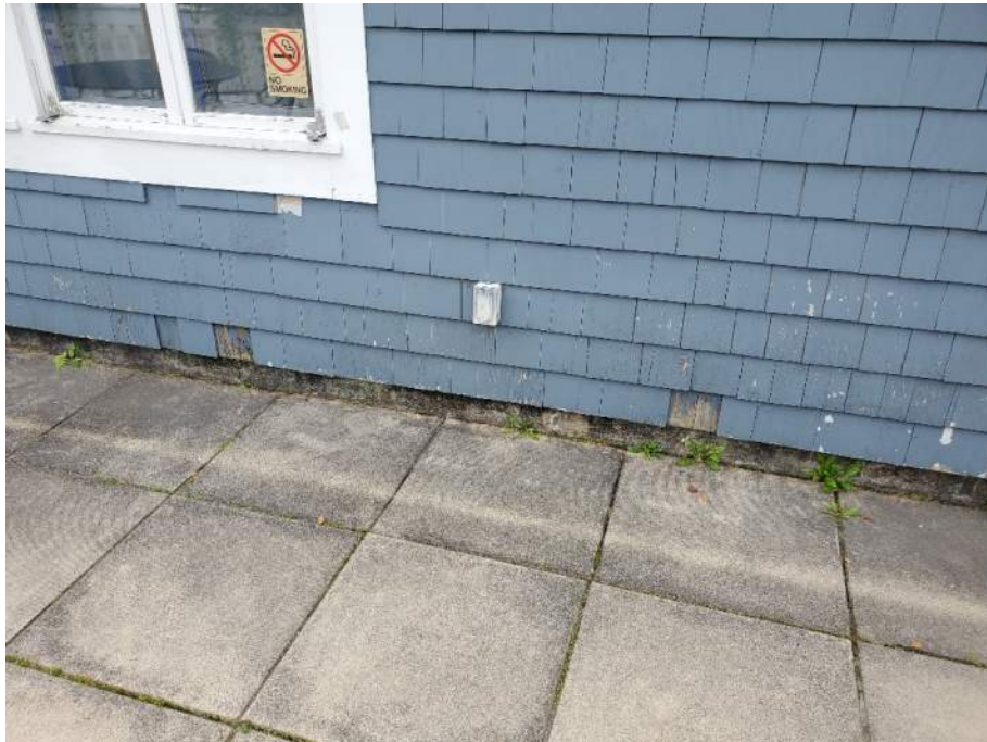
Damaged Siding on North Side
