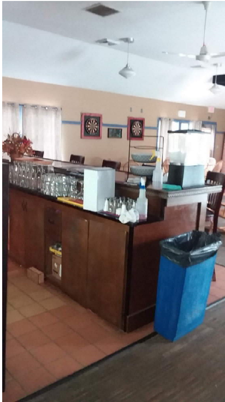
Condition of Finishes on Casework Behind Clubhouse Bar
