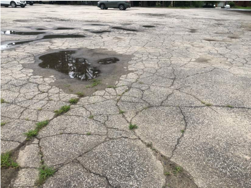
Badly Cracked and Deteriorated Pavement - Typical for All Areas of Parking Lot
