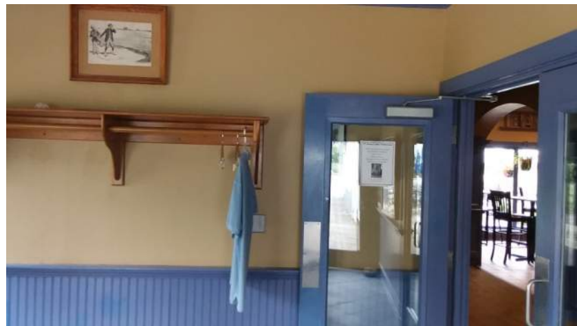
Non-compliant Headroom Clearance in Accessible Path of Travel
