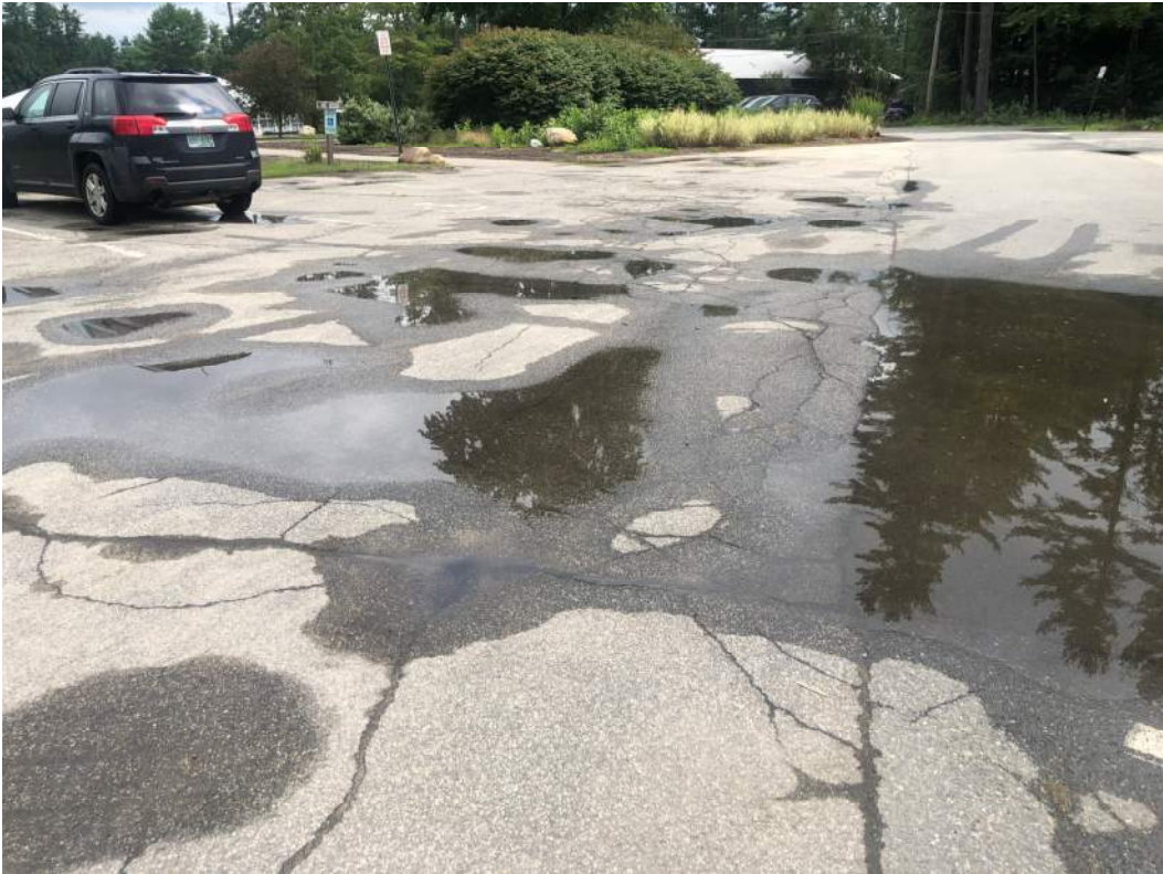
Typical Ponding and Cracked Pavement in Parking Lot – All Areas
