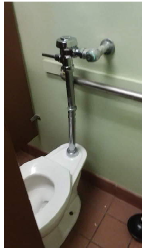
Non-compliant Rear Grab Bar Impairments
