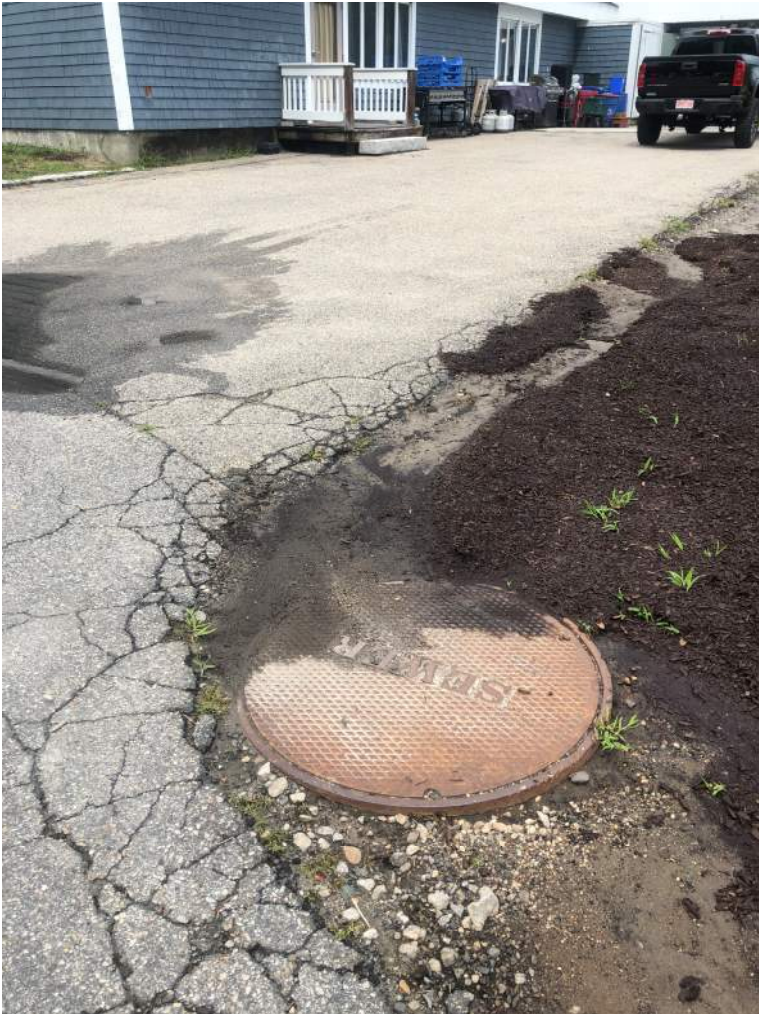
Collapsed Edge of Pavement Southwest of Club House towards Maintenance Building
