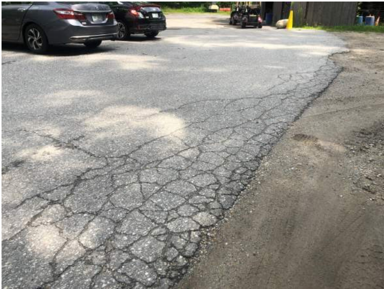
Typical Collapsed Edge of Bituminous Pavement Around Perimeter of Most Paved Areas
