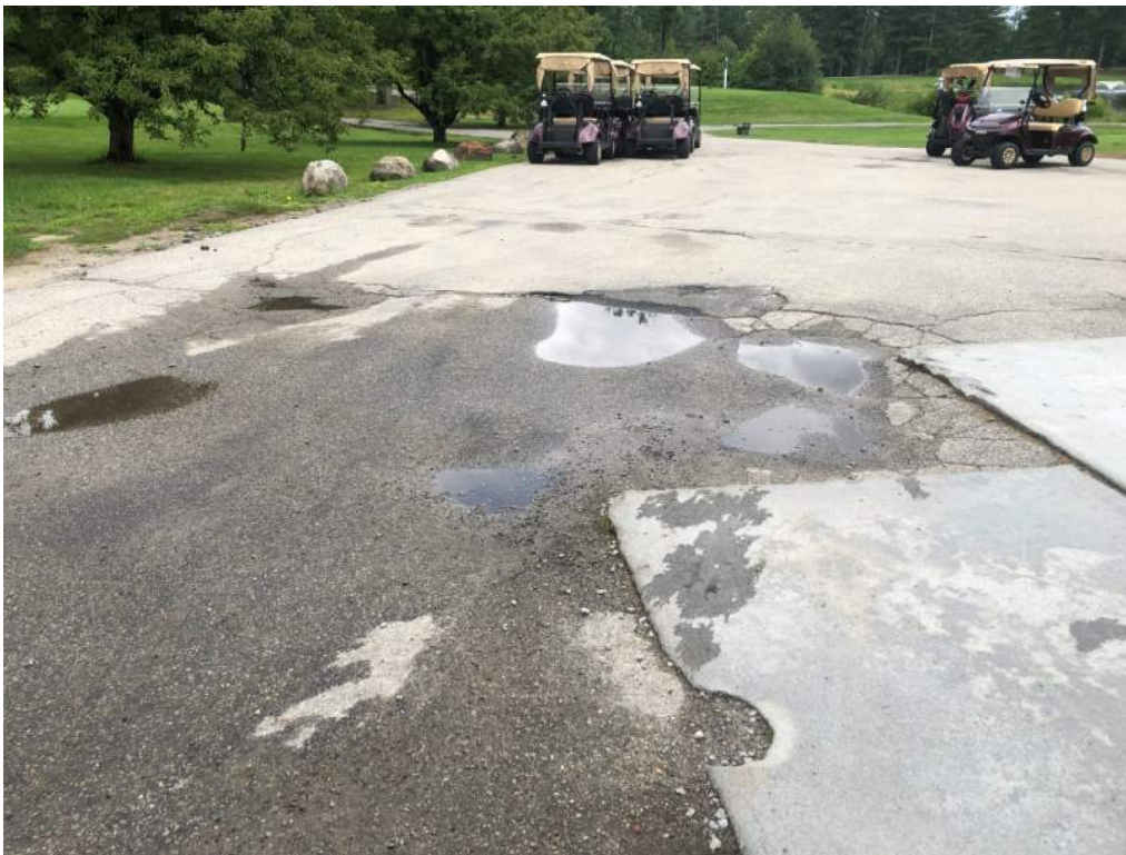
Ponding, Cracked Pavement, Collapsed Edges, Broken Hardscaping, Tripping Hazard – Northeast of Club House
