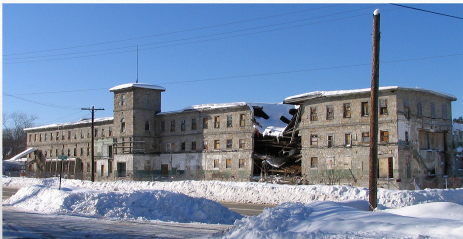
Penacook Mill Collapse 2007
