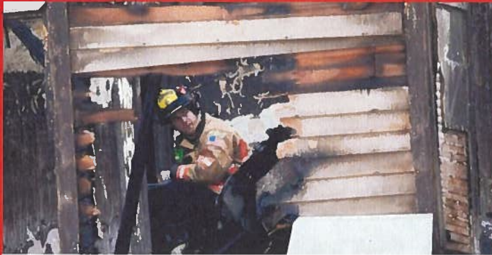
A Rockford Fire Department inspector looks around the second floor of an abandoned home Monday, April 7, 2014, after an early morning fire killed two at the residence in the 400 block of Knowlton Street in Rockford. Rockford Register Star
